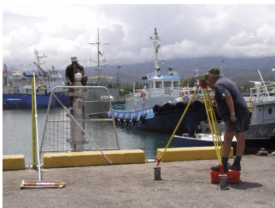
Levelling of SEAFRAME Sensor benchmark. Seated next to SEAFRAME: Andrick Lal, SOPAC. Standing: John Ovenden, NTC. Photo credit: Steve Turner, NTC.
